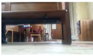
Modern radiant, under pew (360W/m)
