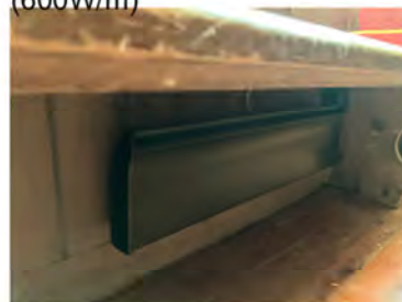
Modern convector, under pew (700W/m)
