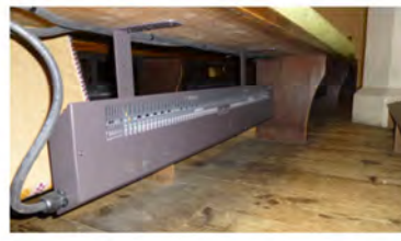
Modern convector, under pew (600W/m)
